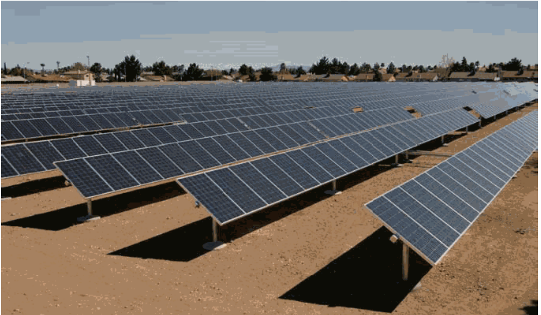
5 MW Solar PV Plant in Andhra Pradesh
