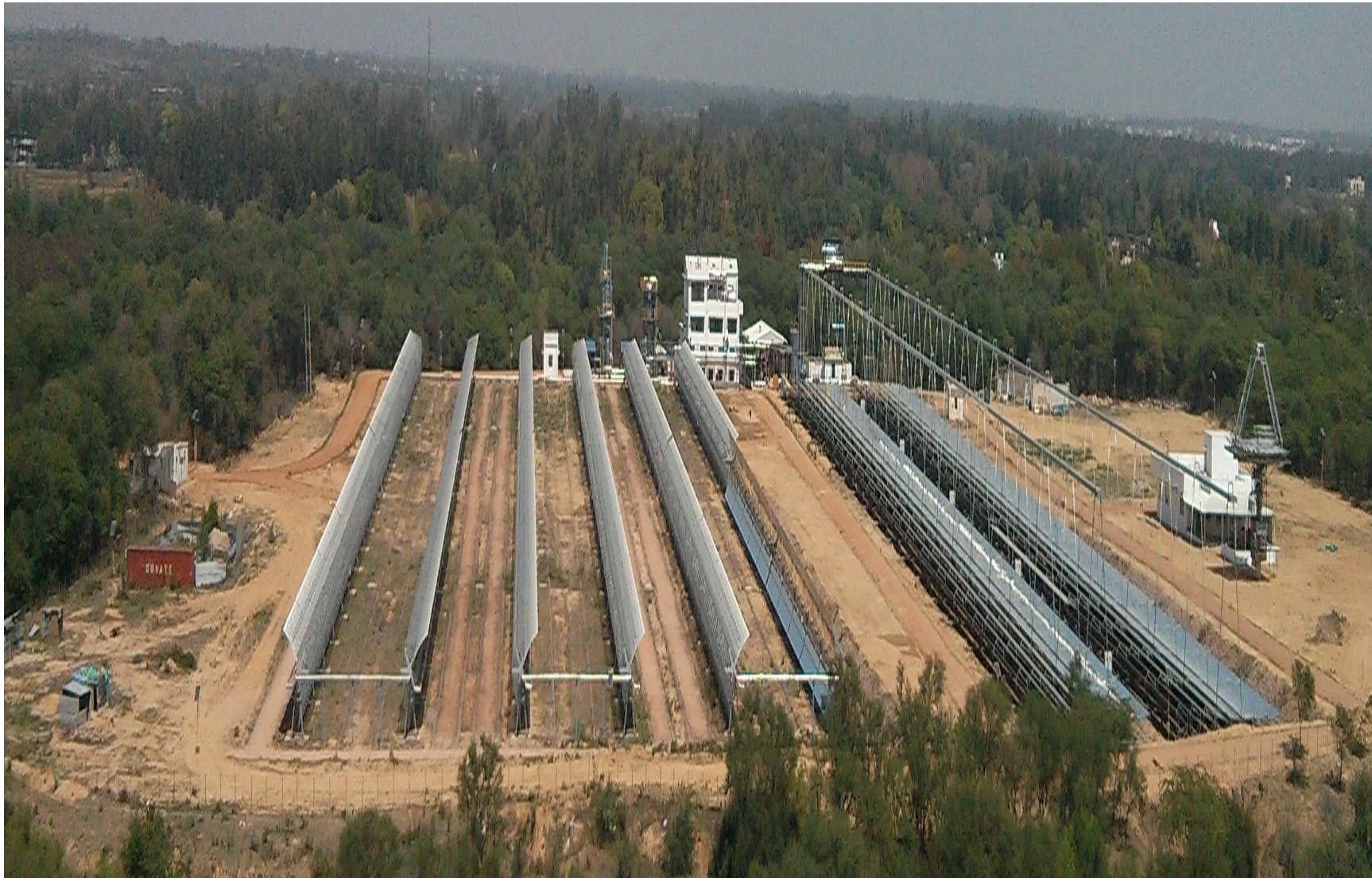
1 MW Solar Thermal Power Plant – Gurgaon, Haryana
