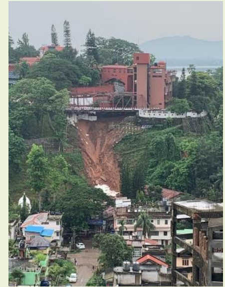
Raj Bhawan Landslide, Guwahati, Assam, 2020
