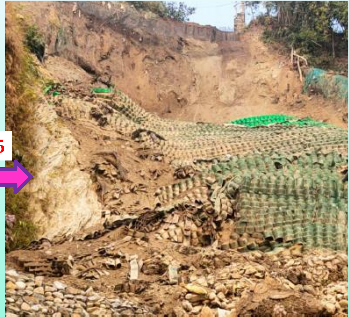
GRS wall: After collapse
