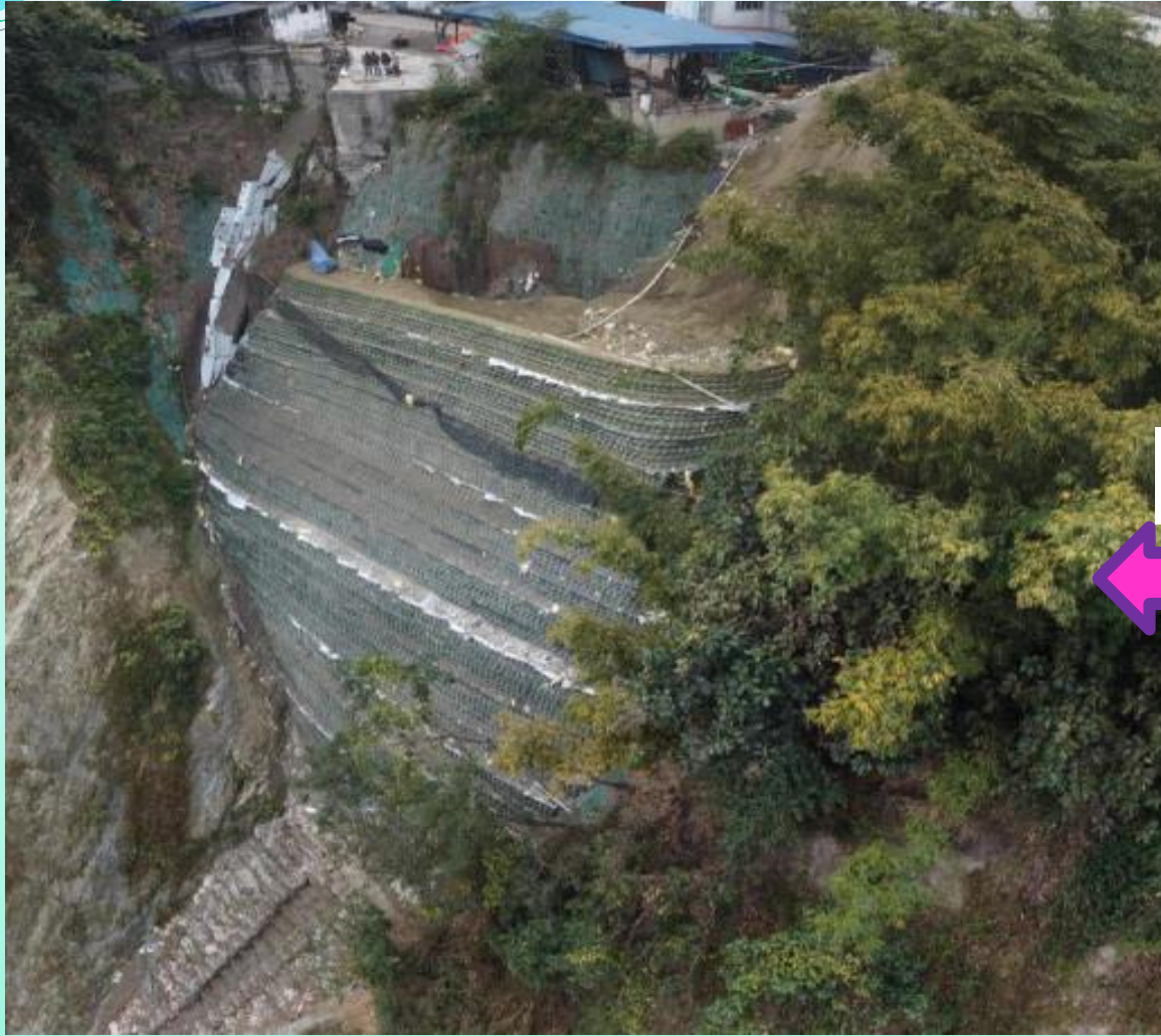
GRS wall: Before collapse (Near completion)
